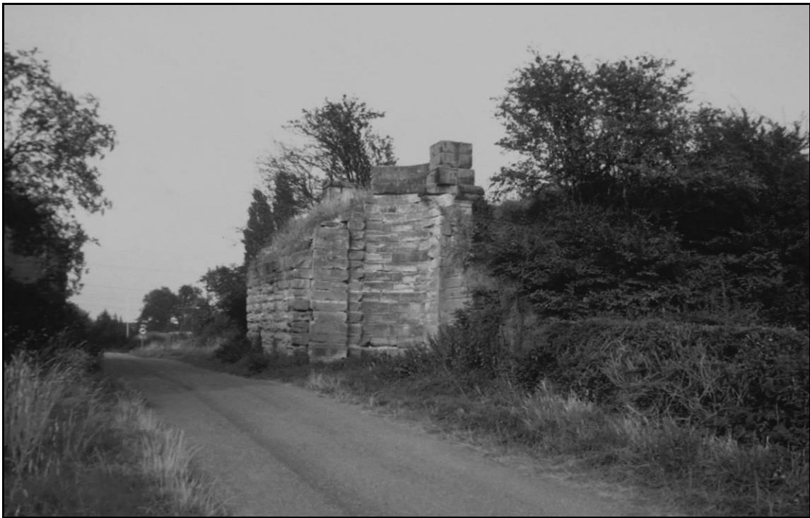
The remains of the bridge which carried the Coleorton railway over Aqueduct Lane, Gelsmoor (known colloquially as Akadoc lane) September 1981, SK407181 looking north-west
