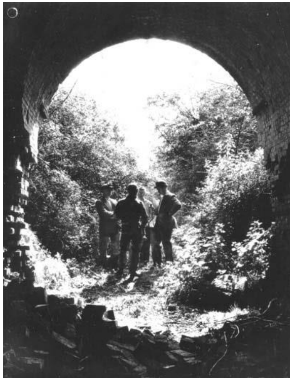
The entrance to the circular brick Pegg's Green Tunnel at St. George's Hill, Swannington which has now been filled in.
