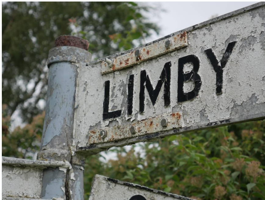
RECENT PHOTOGRAPH SHOWING THE PLATES ADDED SOME YEARS AGO EITHER SIDE OF THE LIMBY FINGER TO SUPPORT A SERIOUS CRACK WHICH HAD DEVELOPED
