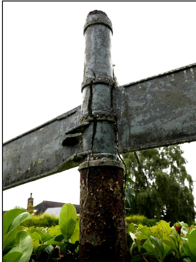
RECENT PHOTOGRAPH TAKEN FROM THE REAR SHOWING THE REPLACEMENT CAST IRON POST
