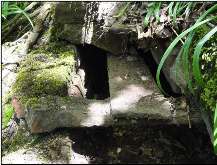
End of circular flue
