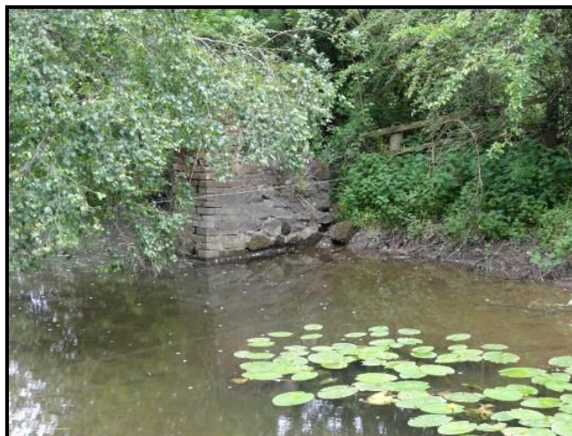
The above photograph is the remains of what we believe to be the stone structure which originally carried the water-wheel. This crossed the brook to the east side of Dimminsdale just before it joins the reservoir.
