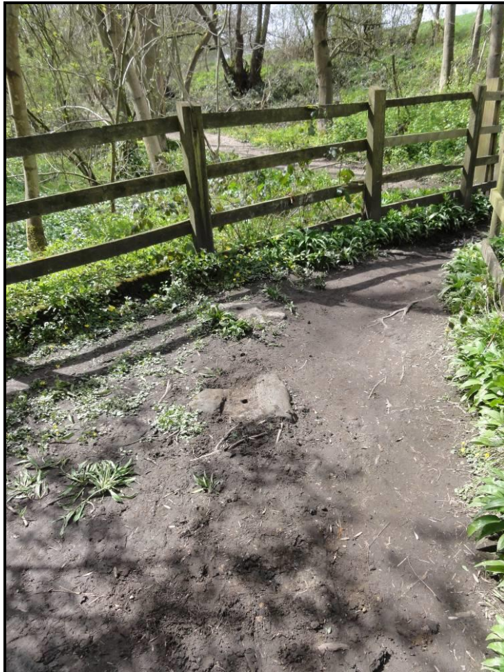
This photograph shows the two sleeper blocks situated in line at 3ft centres on the bridge
