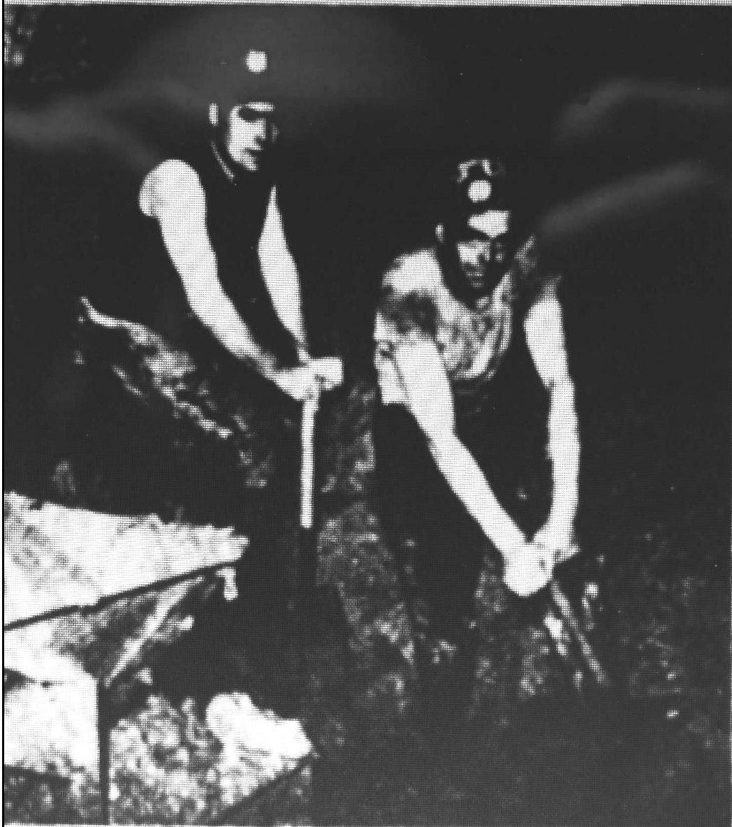
THE BATTLE AGAINST THE MUD goes on at the face of the drift tunnel being constructed at Coleorton.
