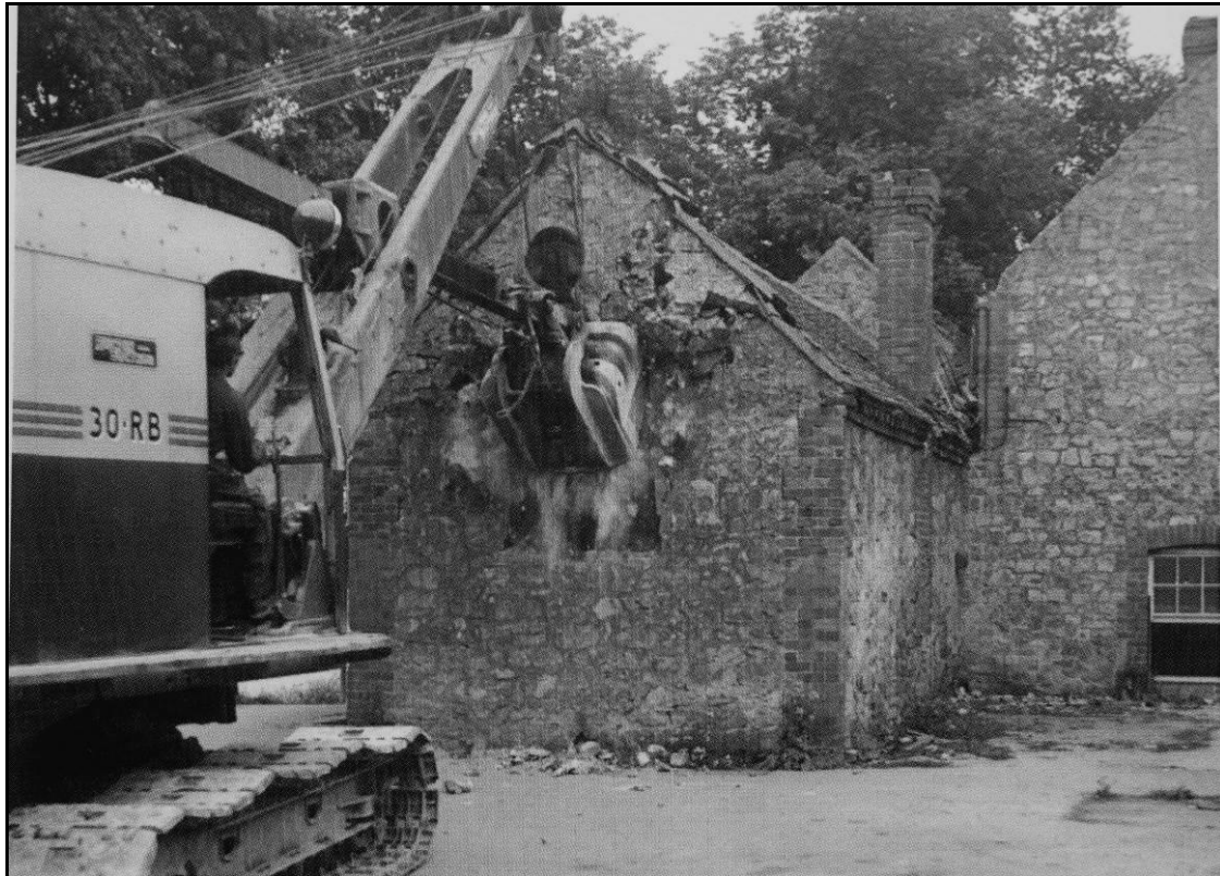
THE END OF THE HOLLY BUSH INN A RUSTON BUCRYUS 30 RB QUARRY EXCAVATOR, EXPERTLY DRIVEN BY DEREK HICKLING, BEGINS THE TASK OF DEMOLISHING THE HOLLY BUSH IN 1965
