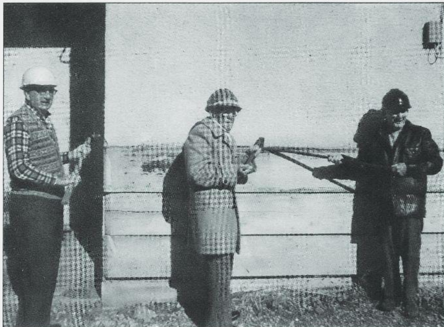
Demolition of Kaleden Co-op Packinghouse. L-R: Clem Battye, Bill King, Jud Findlay. (Courtesy Ron King)
